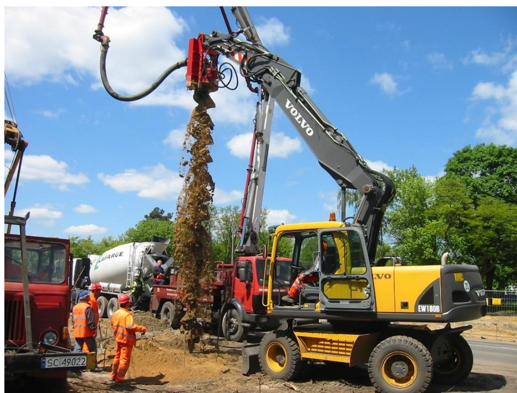
An OWK-3600 type CFA excavator rotating head suspended from a Volvo EW180 wheel excavator – ul. Bukowska, Poznań
