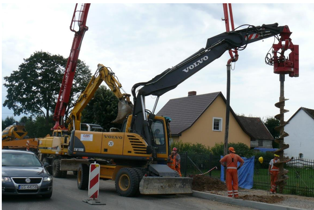
An OWK-3600 type CFA excavator rotating head suspended from a Volvo EW180 wheel excavator – road works on a national road near Słupsk
